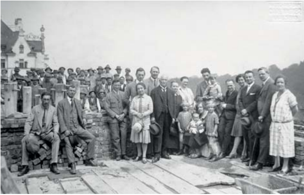
The Gea apartment block under construction, Karlovy Vary, 1928. Rudolf is standing third from right.
